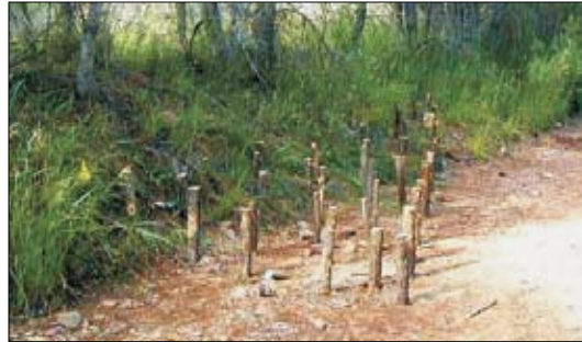
Picket Baffle on Galisteo Creek. (Photo courtesy of Earth Works Institute.)
